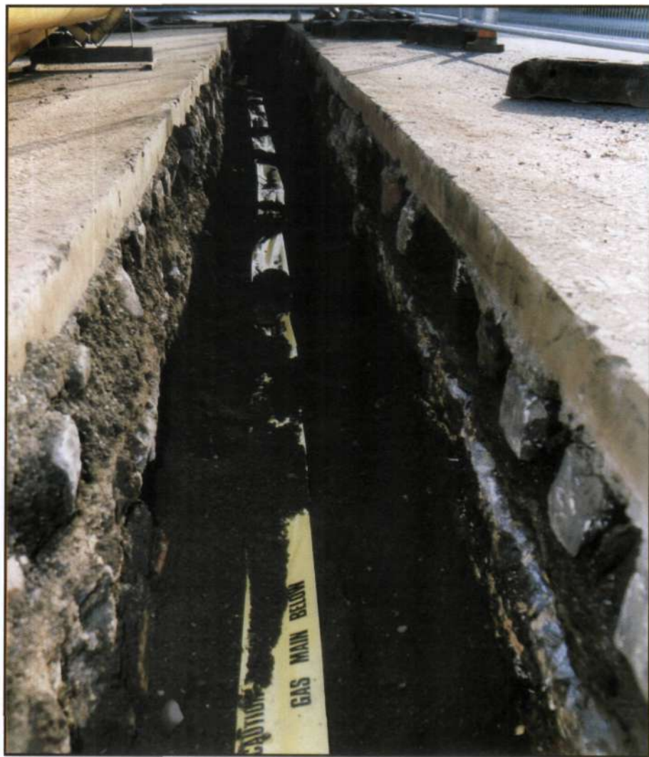
Figure 9 Yellow plastic tape, laid above a gas pipe
